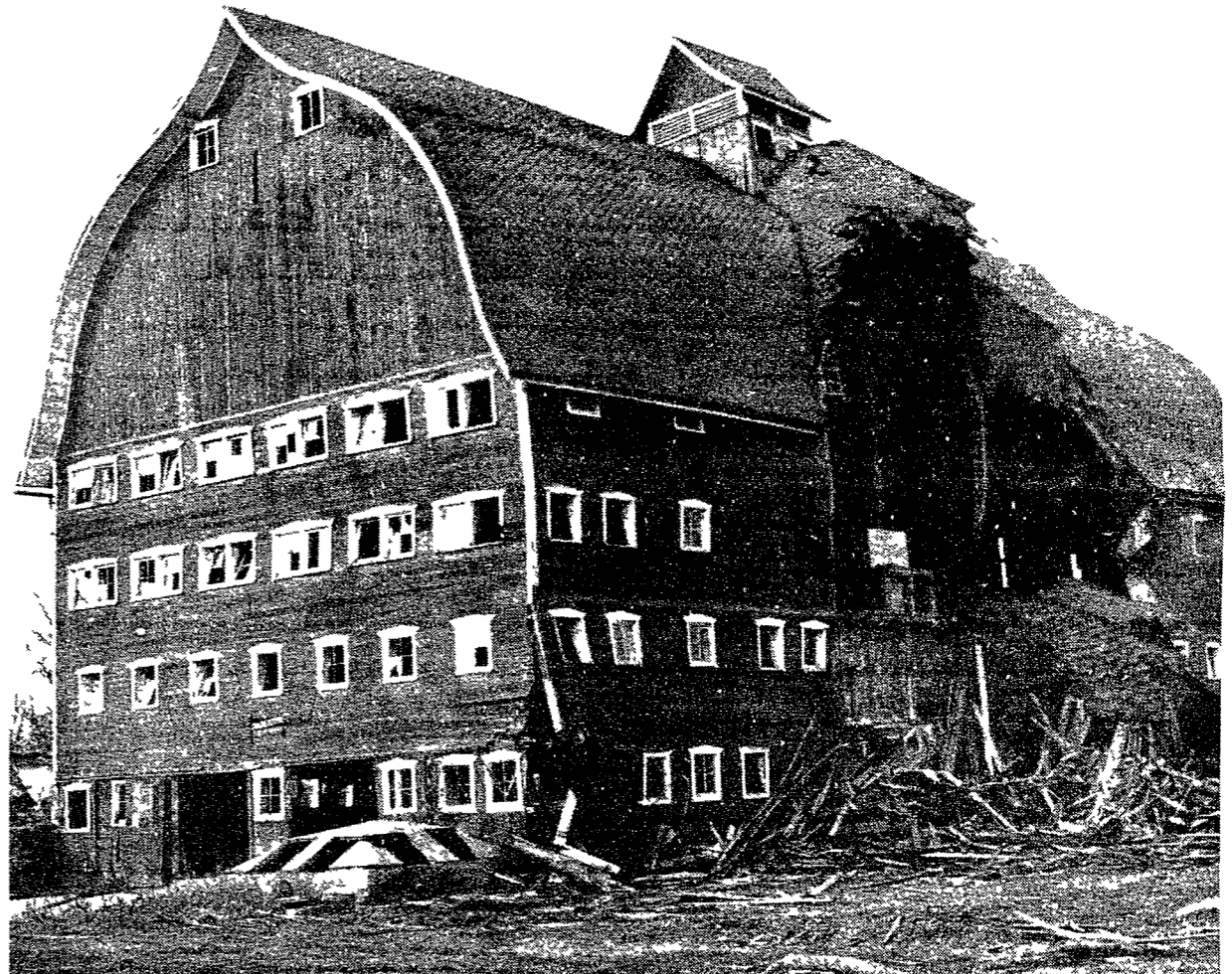
LANDMARK FALLS —Michigan's largest barn fell to progress this week when the historic, cathedral-roofed "big red barn" on the Erwin Apple Farms, Silver Lake Road at Kent Lake Road in Lyon Township, was demolished. The 1907 creation of an MAC (Michigan State University, today) student withstood even a May, 1956 tornado which removed two of three cupolas, but did no other damage to the structure. Edwin Erwin had C. Knox Wrecking of
