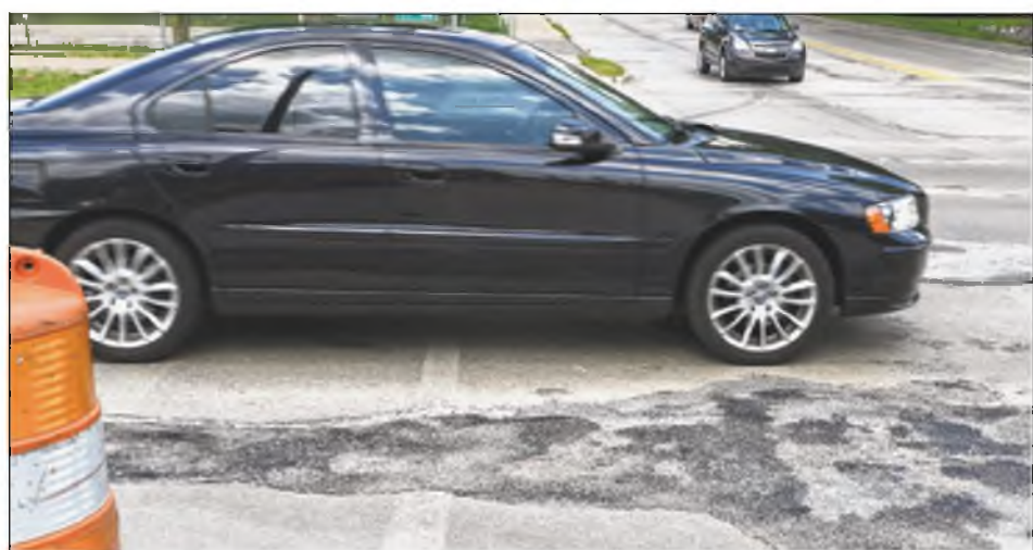
Work should soon commence on the renovation of Eight Mile Road between Center and Meadowbrook on Northville and Novi's border. JOHN HEIDER | STAFF PHOTOGRAPHER
