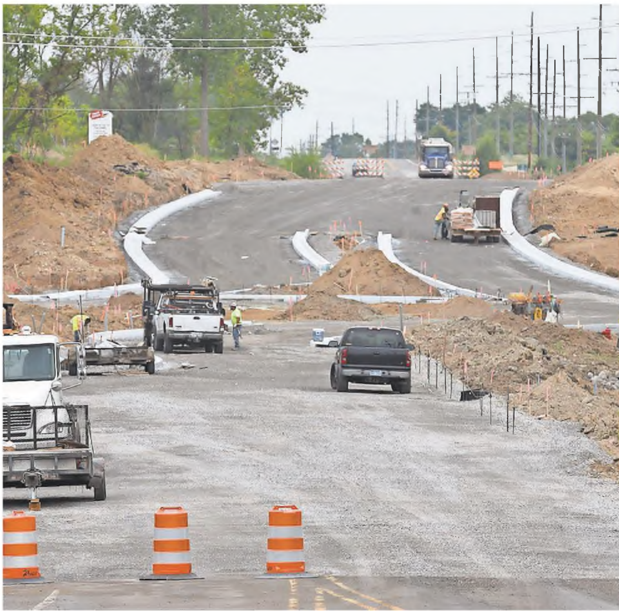
Work continues Aug. 28 on the roundabout project on 10 Mile at Napier roads in Lyon Township. Traffic will be closed at the intersection until early October as a new intersection is created, making transit, especially along Napier, much easier. 10 Mile Road, west of Napier, is being leveled a bit to improve sight distances.
