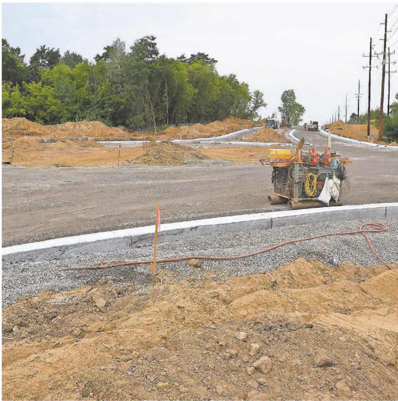
A ground-level view of the roundabout taking shape at 10 Mile and Napier.
