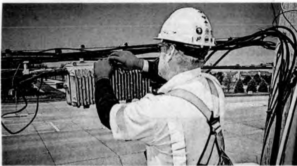
A technician working on behalf of Comcast installs network infrastructure. The company recently completed a $4 million expansion in South Lyon. SUBMITTED
