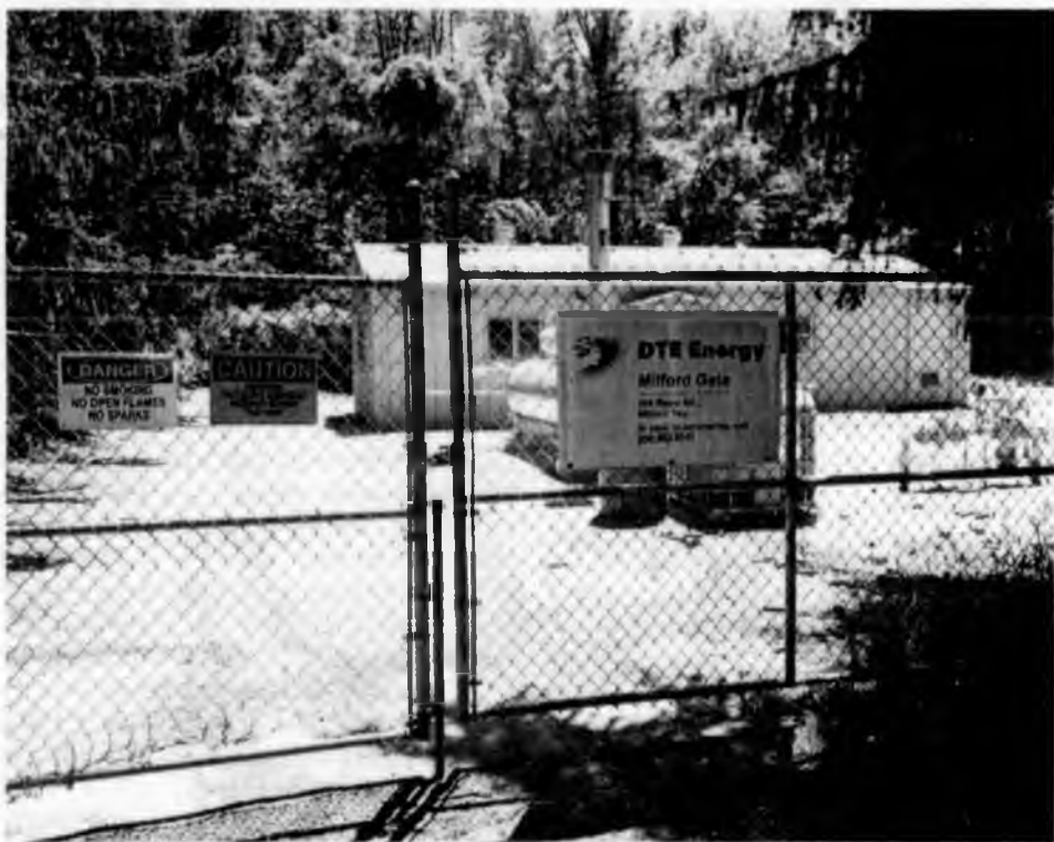
This DTE gas pipeline substation is a quarter mile from Ouellette's home.
