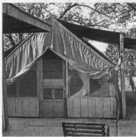
The green military-style tents at Camp Dearborn in Milford have been deemed a "critical infrastructure failure."
