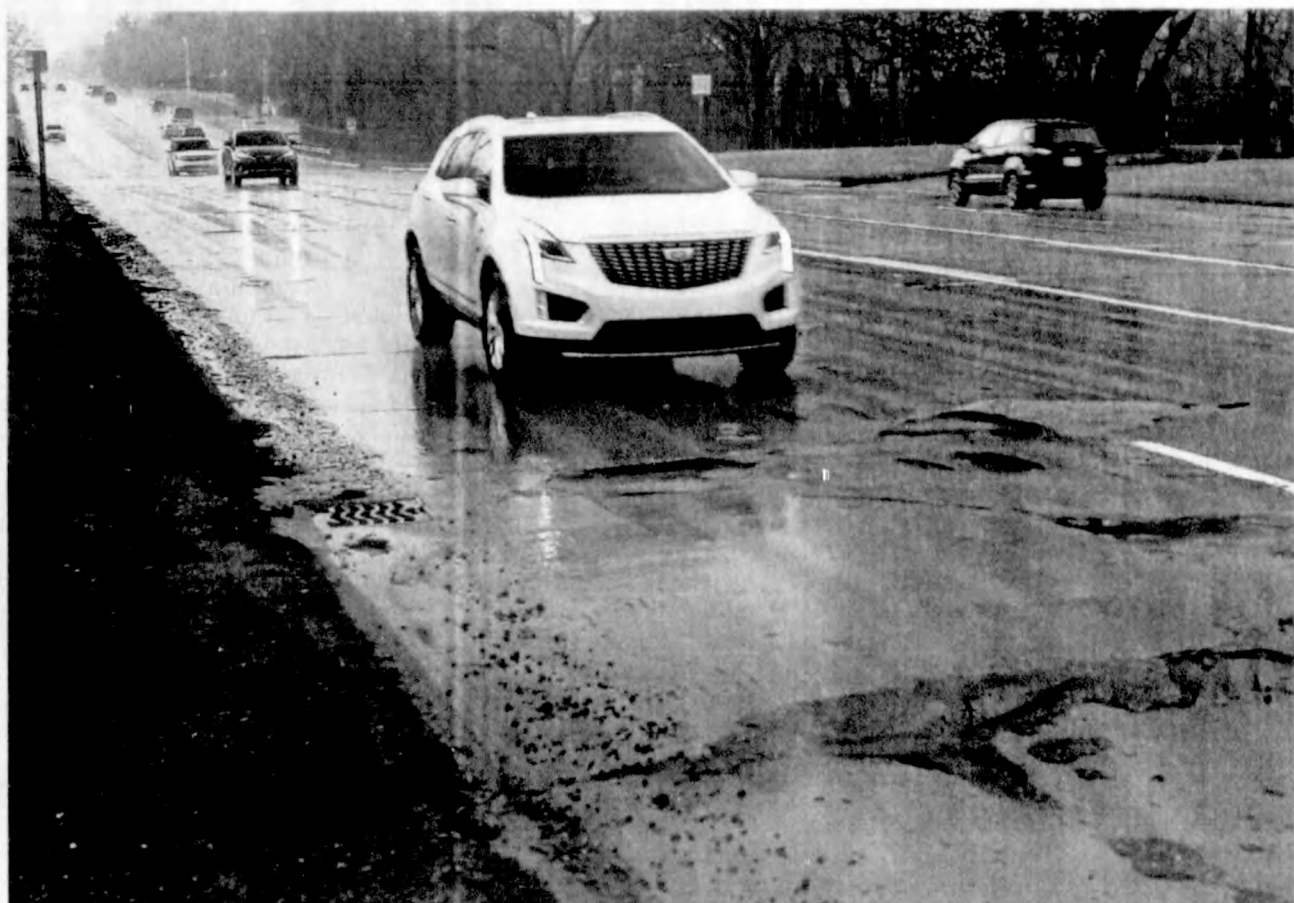
Vehicle drive along Eight Mile near Meadowbrook on the Novi/Northville Township border. The road, which has plenty of patches, hopes to see construction in the future. DAVID VESELENAK/HOMETOWNLIFE.COM
